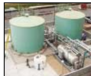
In place and doing its job: a complete U 2 A system operating at Huntington Beach, California
