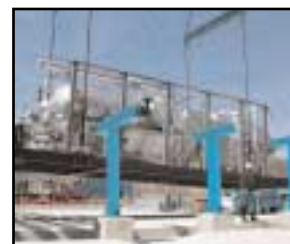
The heart of the system: 4,000 lb/hr U 2 A hydrolyzer is lowered into place in West Virginia. This versatile process has been scaled from 2 lb/hr to over 10,000 lb/hr capacity in field installations.
