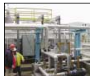
Hydrolyzer feed pump maintains constant solution level in the hydrolyzer.
